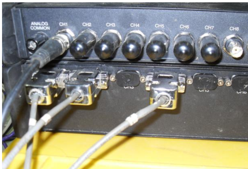
Figure 19. The back view of the data acquisition system after RAM Test wires are plugged in, general procedure to prepare RAM Test step 1
